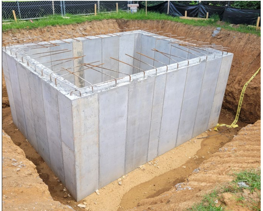
Surge tank for the new Douglass Pool
