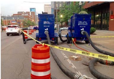
Above ground: bypass pumps keep the system fully operational
